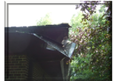
Eavespout on headquarters building damaged by storm
